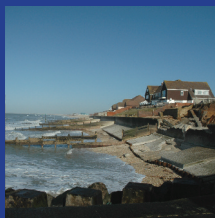
Damaged coastal defences in the United Kingdom.
