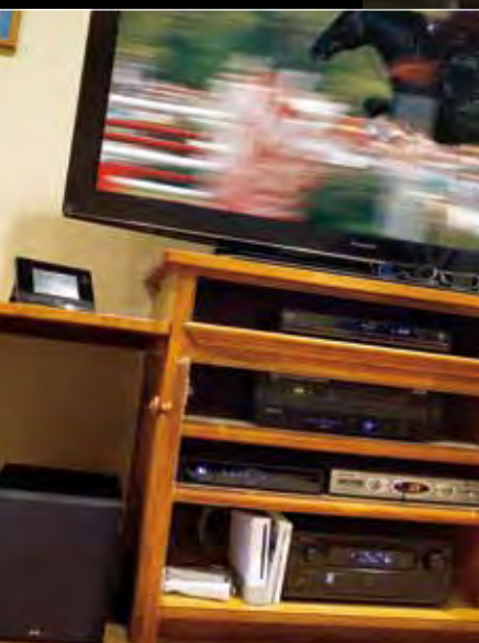
Below: The game room. Complete with a 3D HDTV, Wii gaming system and AMX control.
