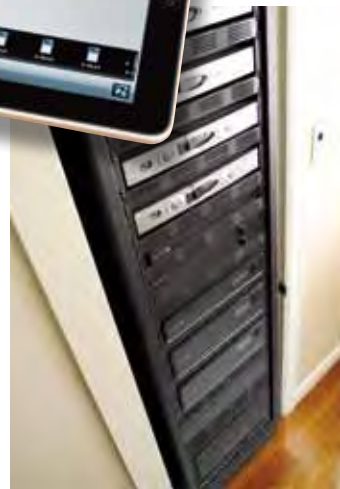
The audio and video components for the home are housed in two racks that were built and outfitted by Magnolia. Control is made easy with the Control4 iPad app.
