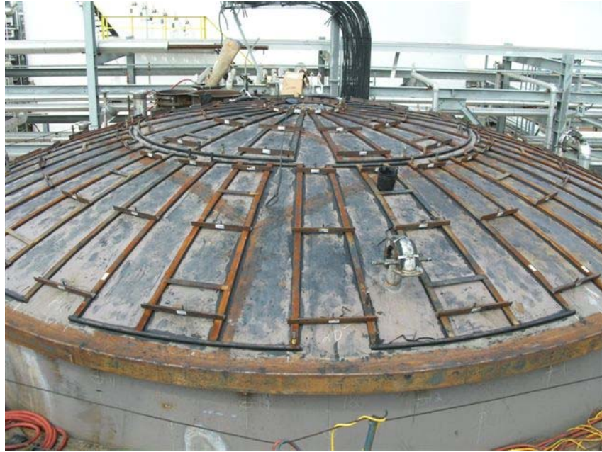
Figure 4: Example ControTrace tank roof heating
