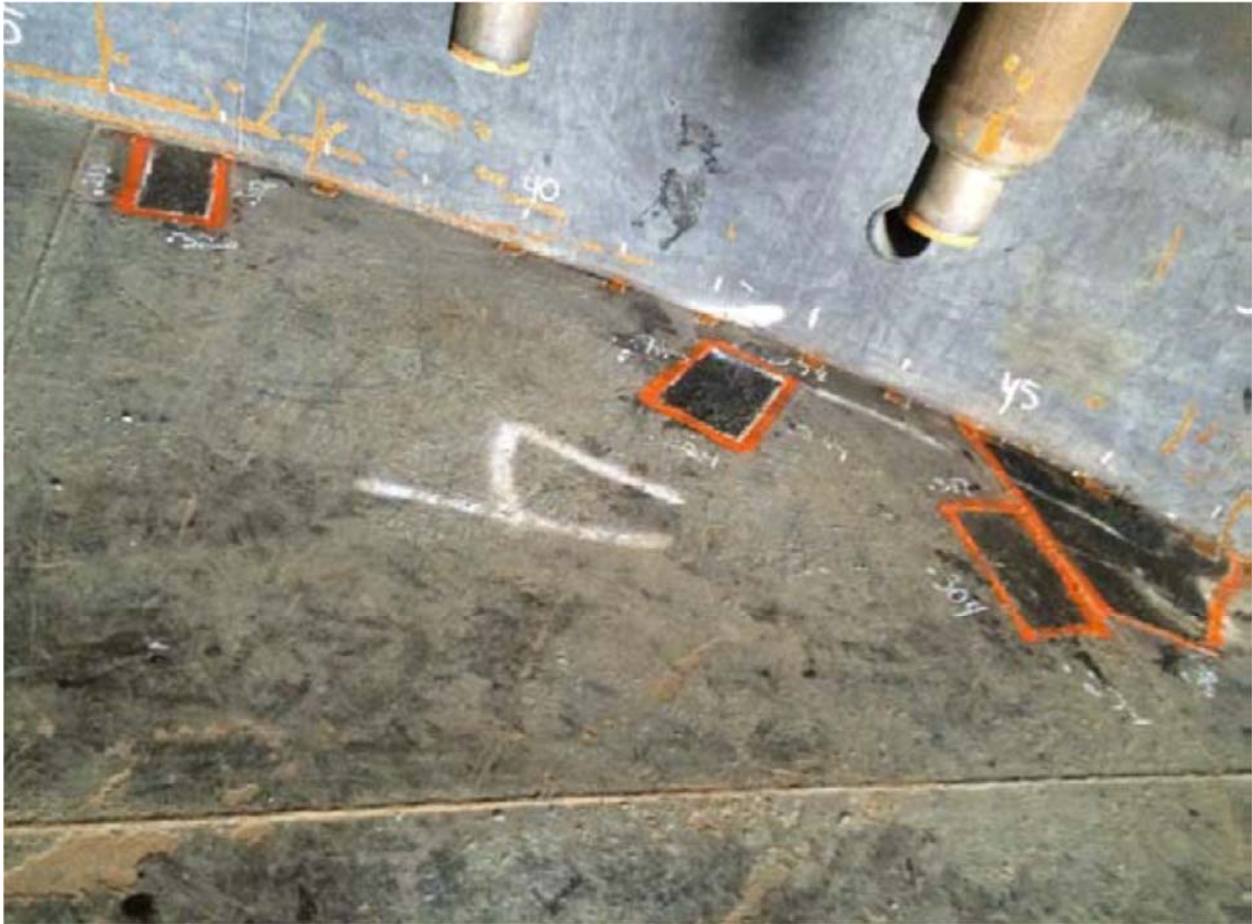
Figure 13: Typical tank floor surface with bottom-up corrosion near perimeter; boxes mark UT measurement locations
