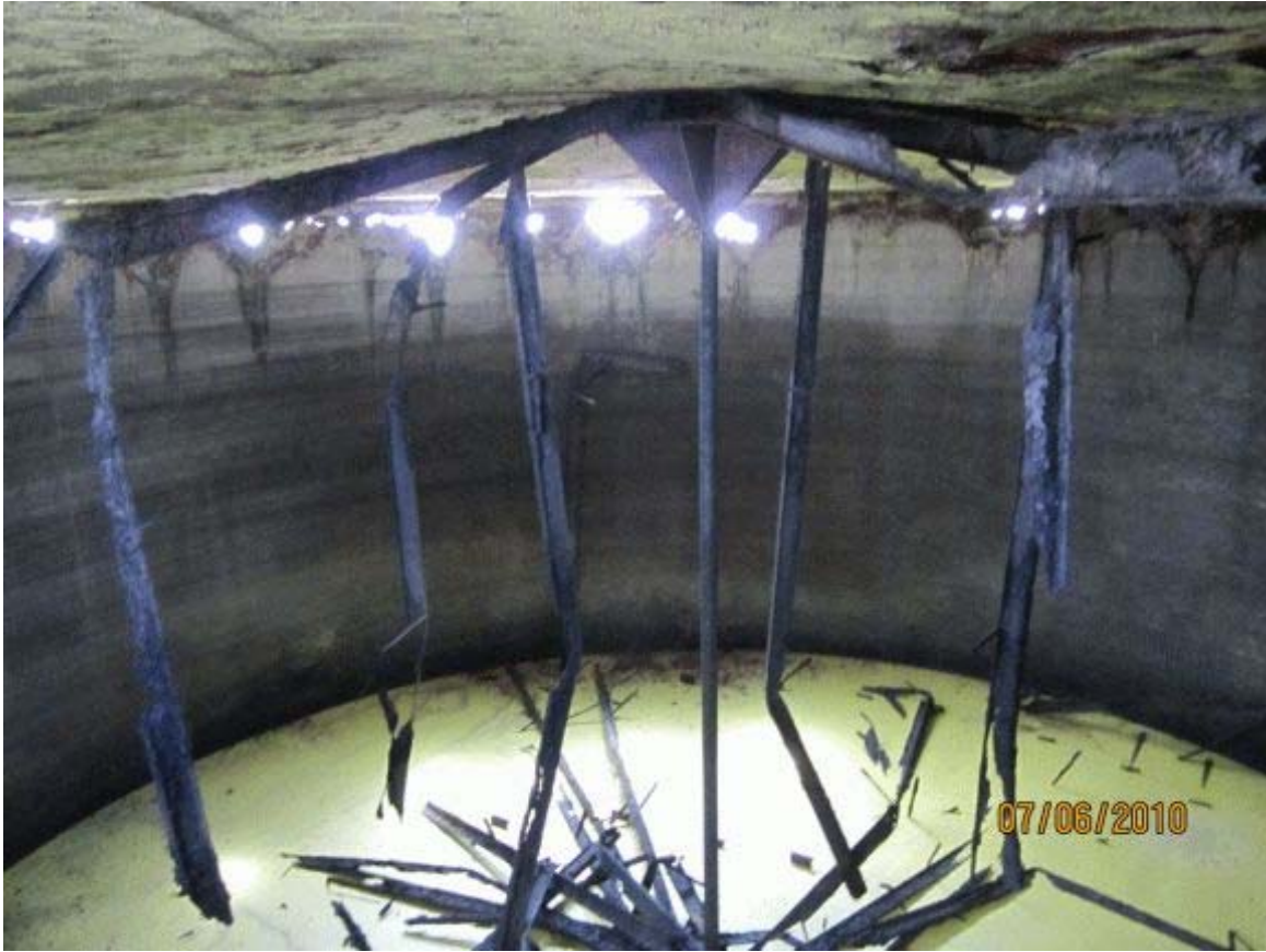
Figure 3: Example sulfur tank structure corrosion
