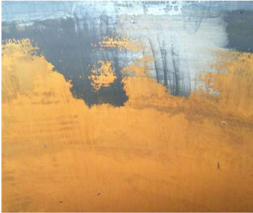
Figure 11: Typical interior shell/roof surface with light coating of rust
