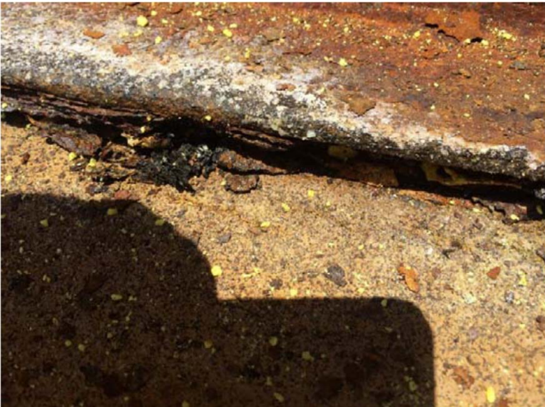
Figure 10: Corrosion and scale under tank chime
