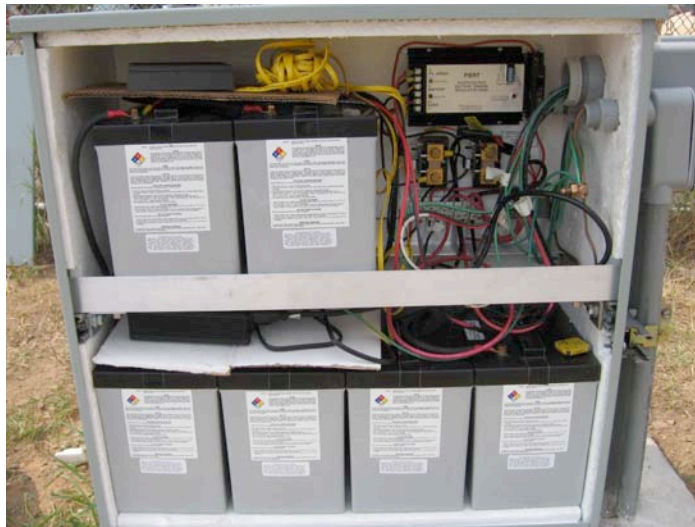
Figure 9: Cabinet for Holding Batteries and Control Units.
