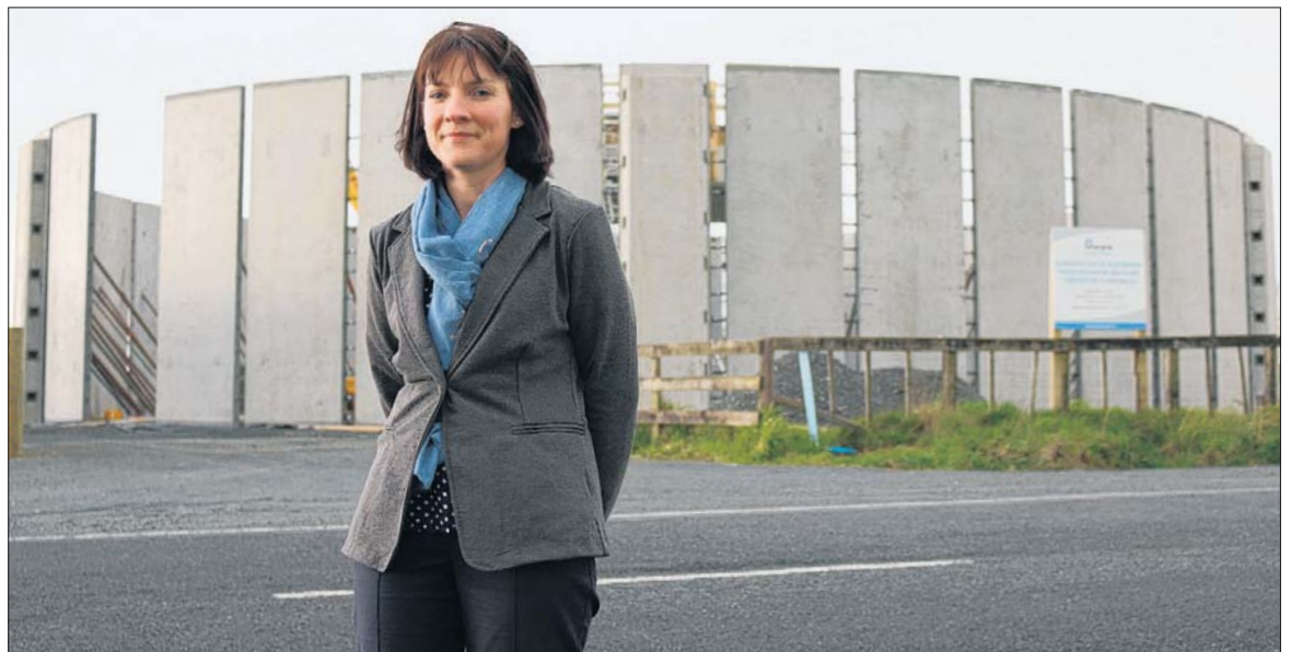
WAIPA water service delivery manager, Lorraine Kendrick, in front of Te Awamutu's new water reservoir being constructed on Frontier Road. The reservoir will come 'on stream' early next year and hold 6,000 cubic metres of water. It will provide extra capacity during times of peak water use and for fire fighting, but will not eliminate the difficulty Council has complying with abstraction consents at Te Tahī Road in summer.
