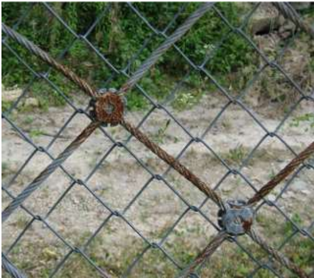
Picture 2.5 Corrosion problem of wire rope nets (cross clips and rope wires do often have no sufficient zinc coating and may rust rather soon)
