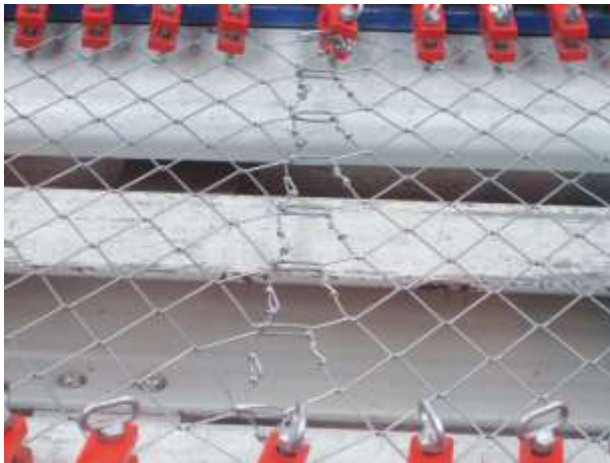
Picture 5.26 Condition right before the collapse of the high-tensile steel wire mesh
