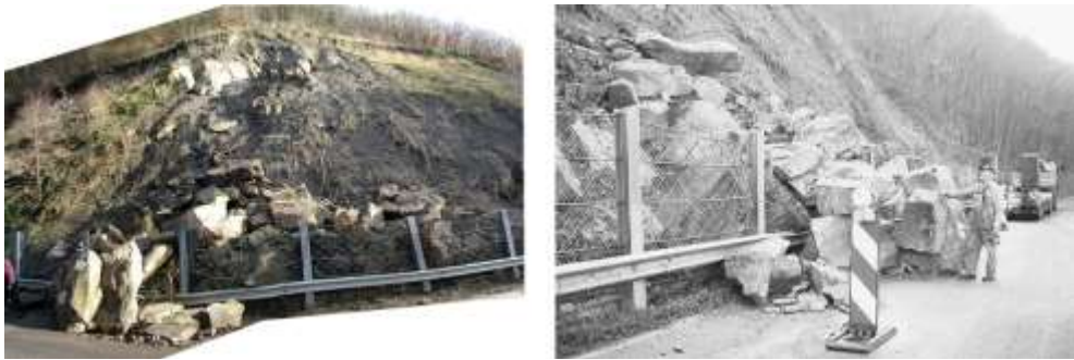
Picture 11.10 Slide, causing the temporary closing of the regional road
