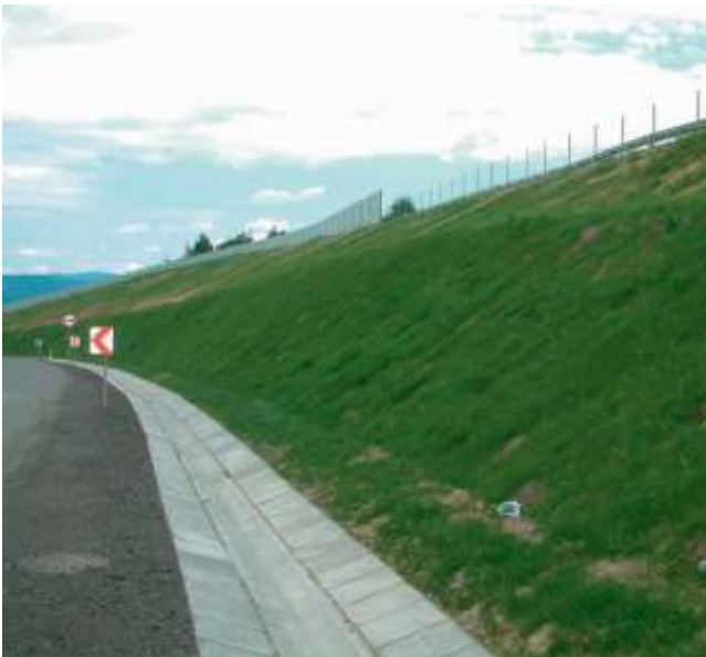
Picture 11.39 Picture of the slope three month after completion of installation work
