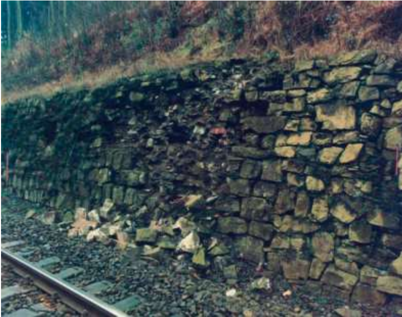
Picture 11.65 Old, partly broken brick wall at railway line
