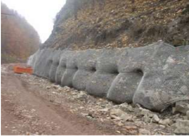
Picture 5.32 Slope stabilization system made with traditional steel wire meshes (chain-link, 50 \times 50 mm, 4.6 mm wire diameter). Nail distance was chosen too large and consequently, large deformations of the wire mesh occurred in short time.
