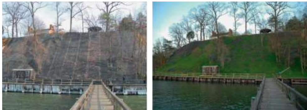
Picture 11.64 TECCO® slope stabilization USA (left during installation; right several months after completion of installation)
