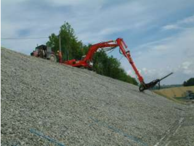
Picture 11.30 Drilling process from with access from the top of the slope
