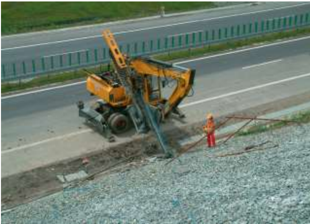
Picture 11.31 Slope under nailing works. Partially covered with crushed stones due to local failures of the slope surface
