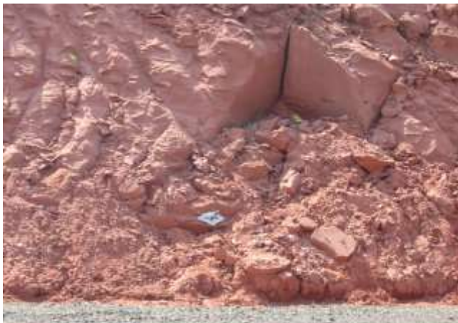
Picture 11.21 Wedge-shaped failure due to relaxation
