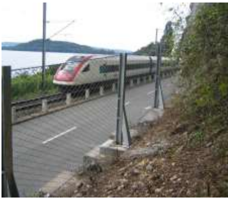
Picture 5.1 Rockfall barrier with high-tensile steel wire mesh
