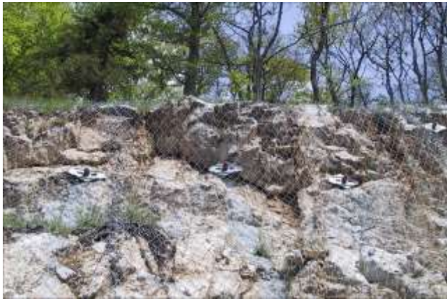
Picture 10.14 Positioning of principal spike plates in areas of hollows (in the terrain surface)
