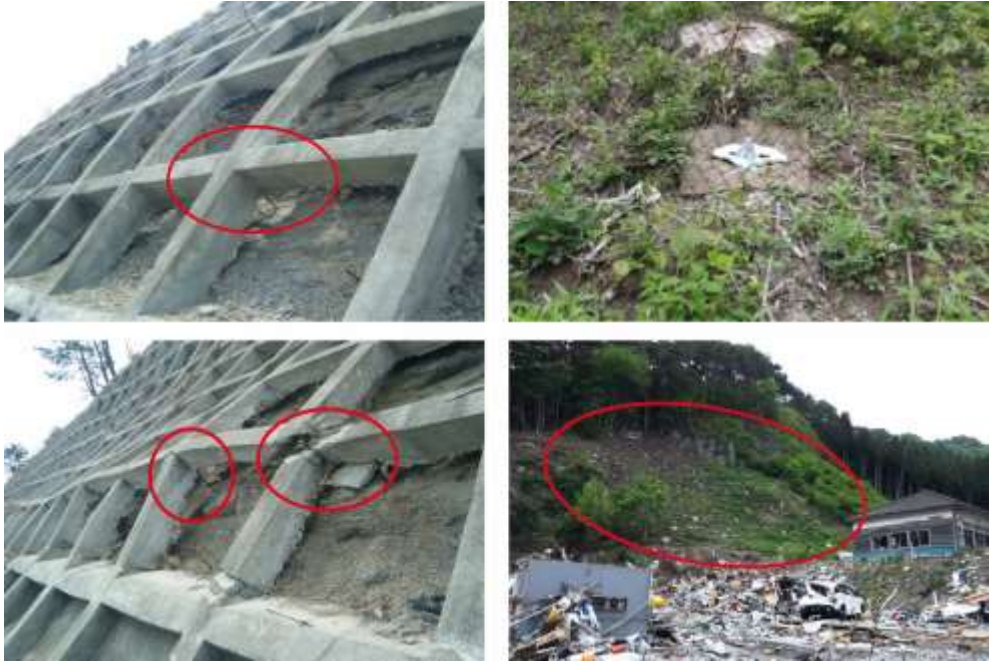
Picture 11.69 Slope stabilizations in Sendai area (close to Fukushima, Japan) after the heavy earthquakes in March 2011. Left pictures show a failed concrete slope stabilization due to earthquake influences. Right pictures show a TECCO® slope stabilization that resisted all earthquake influences perfectly without any damages.
