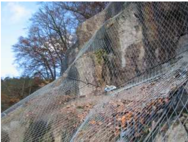
Picture 11.14 Location of nail and spike plate in deep point of the slope
