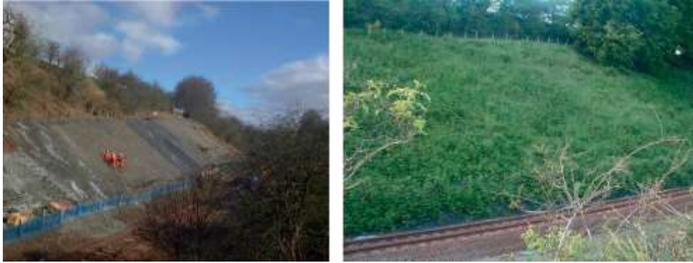
Picture 11.63 TECCO® slope stabilization at Neilston, UK, Railway cutting near Glasgow (left during installation; right several months after completion of installation)
