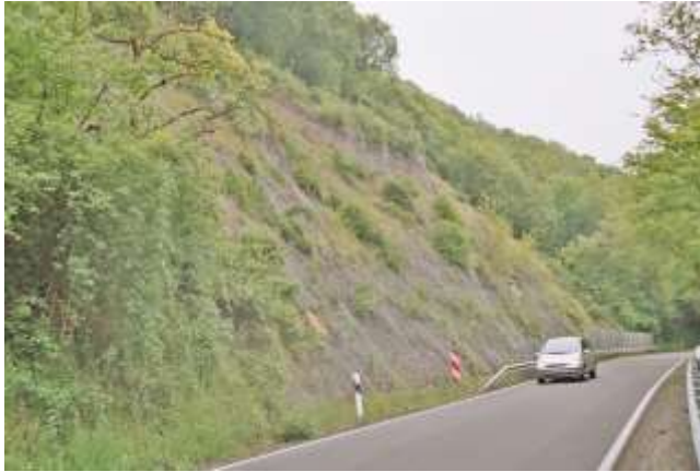
Picture 10.22 Slope stabilization using high-tensile steel wire meshes in combination with nailing (TECCO® System)
