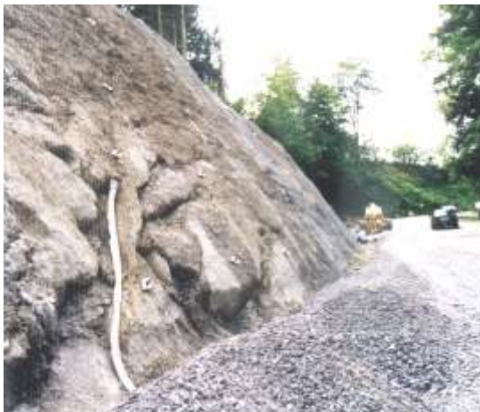
Picture 10.16 Drainage hose to drain arising hillside water
