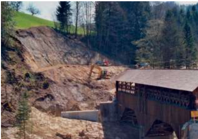
Picture 11.1 Cut slope at the bridge of Anzenwil during the construction phase
