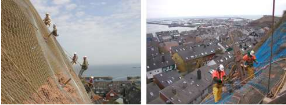
Picture 11.17 Left: Installation of TECMAT and high-tensile steel wire mesh Right: Drilling processes with light weight equipment
