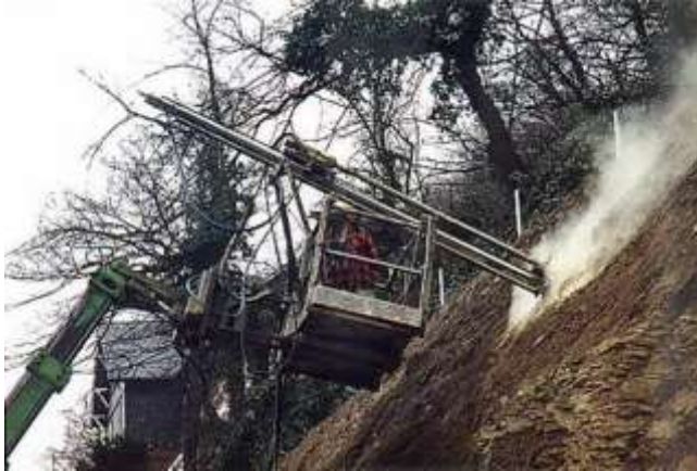
Picture 10.11 Depending on local terrain conditions, drilling work can also be carried out from a small crane platform or lifting platform
