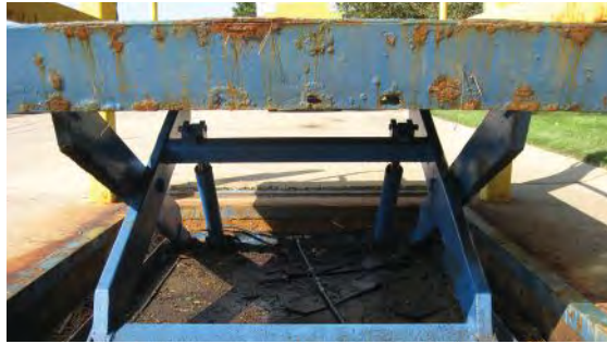
Without the need for pits, surface-mounted lifts are becoming more popular—but they still require regular cleanings and maintenance.
