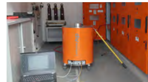
Partial discharge diagnosis on a medium voltage cable
