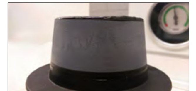
Signs of PD on a substation bushing
