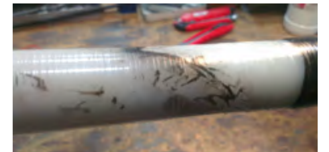
Signs of partial discharge on a defective termination
