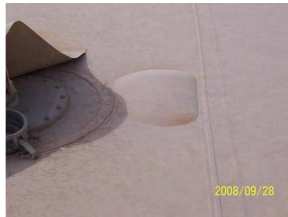
Figure 11. Example of blister on seam
