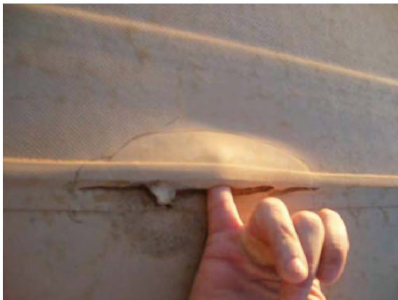
Figure 14. Example of a seam separation (no leak)
