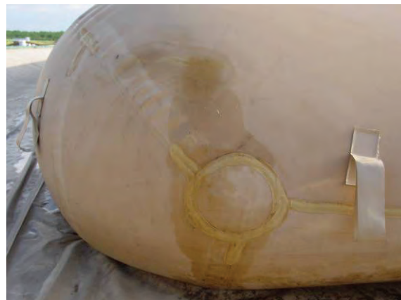
Figure 4. Example of Class II leak
