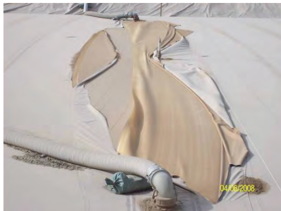
Figure 13. Example of delamination
