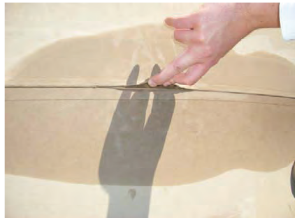
Figure 15. Example of seam separation (leak)
