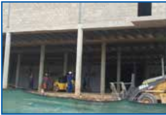
Concrete Frame Structures [Columns & Beams] Shopping Centres; Schools; Multi-storey Residential; Commercial etc.
