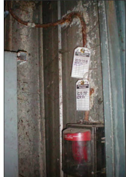
Photo 9-3: Fire detection and alarm systems inside organic processing facilities are particularly susceptible to damage from corrosion © CH2M HILL
