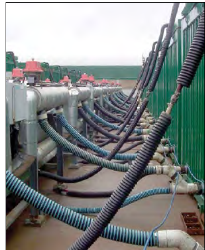
Photo 5-22: Each static container is attached to a central air system using flexible hoses © CH2M HILL
