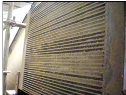
Photo 15-1: Dust can quickly clog radiators on windrow turners and other equipment, and lead to overheating © CH2M HILL
