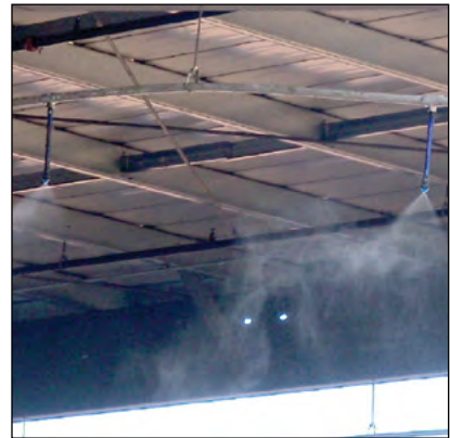
Photo 15-2: Roof-mounted and directional misting systems installed inside buildings and around equipment are effective at controlling dust levels © CH2M HILL
