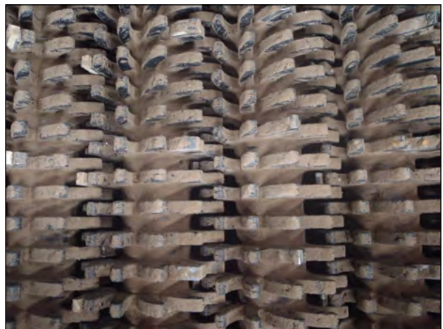
Photo 11-8: Top view of a series of shafts with rubber stars in a star screen (material flow is from left to right across the deck) © CH2M HILL
