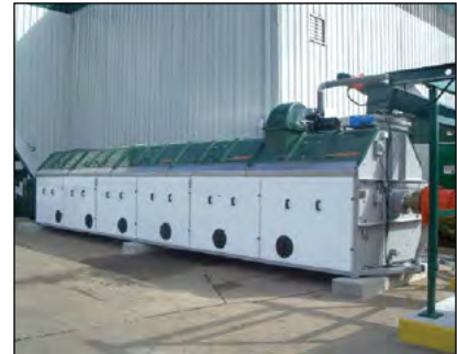
Photo 5-24: Agitated container system © CH2M HILL
