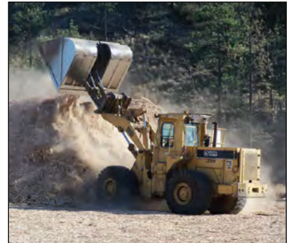
Photo 11-2: Front-end loader equipped with a roll-out bucket, which significantly enhances reach and versatility © CH2M HILL
