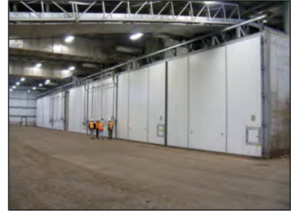
Photo 5-17: Enclosed tunnel composting system © CH2M HILL
