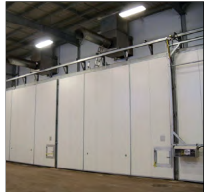
Photo 5-18: Closeup of tunnel door system © CH2M HILL
