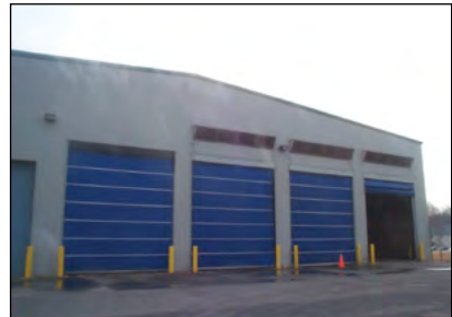
Photo 10-4: Rapid-cycle rubber overhead doors used at a composting facility © Scott Gamble
