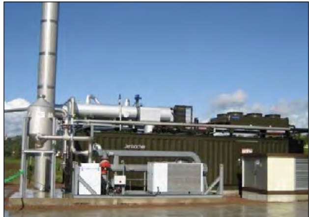
Photo 7-1: Package CHP system © CH2M HILL
