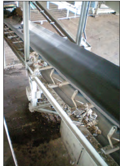
Photo 11-15: Conveyor belts provide efficiencies in moving large quantities of materials within a processing facility © CH2M HILL
