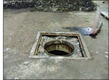
Photo 10-8: Underground sumps and tanks are commonly used to collect and store high-strength leachate © CH2M HILL
