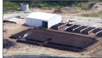
Photo 5-10: A mass bed system in the process of being turned; note turner location at bottom left of the pile and aisle created behind the turner © Lenz Enterprise Inc.
