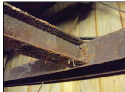
Photo 9-12: Corrosion has proven to be one of the most challenging design issues for the organic processing industry © CH2M HILL
