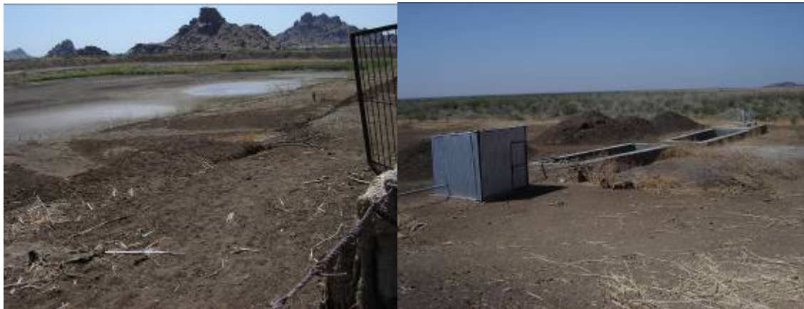
Figure 6. Dry hafir with its slow sand filtration system
