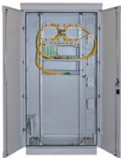
Street Cabinet PU-10 with FTTX equipment
