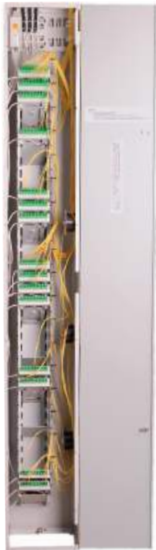
Central office cabinet PSU-300/432
