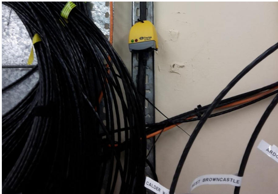
Figure 22: Tinytag located in East Kilbride South substation
