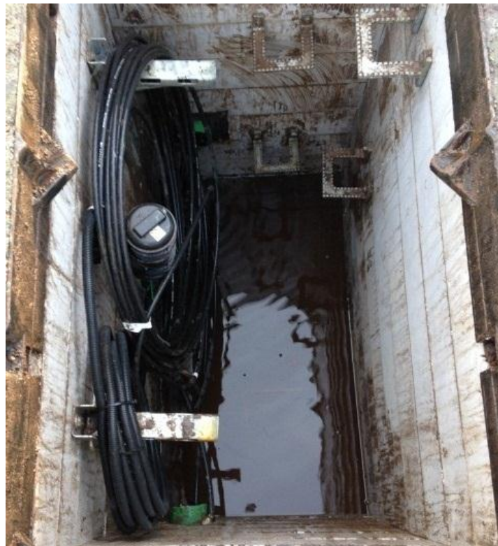
Figure 10: Chamber and DTS fibre joint box
