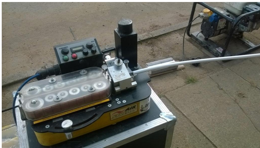
Figure 12: CBS Airstream blowing head (location: EKS substation)
