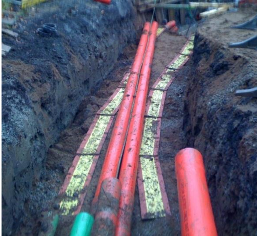
Figure 6: Micro-duct is placed on the top of the two cable ducts before fitting the third cable duct
