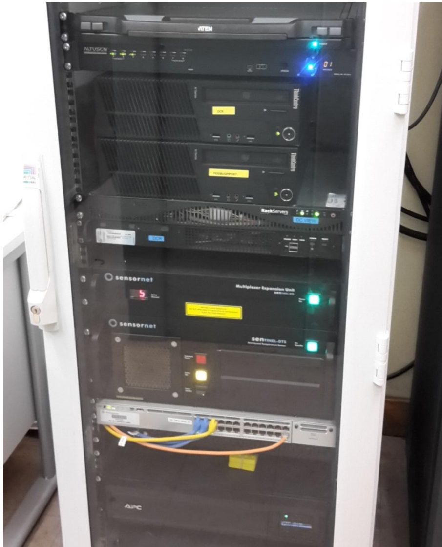
Figure 20: DTS system cabinet at EKS substation
