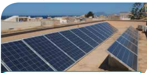
Solar PV system installed on the roof of the Casa Comunale, Favignana, Italy
