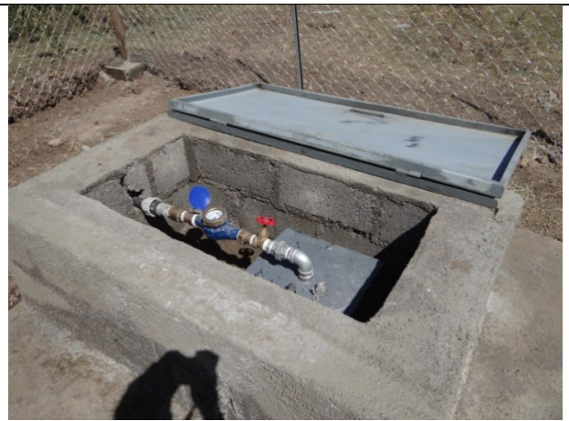
Well head with gate valve, meter and check valve
