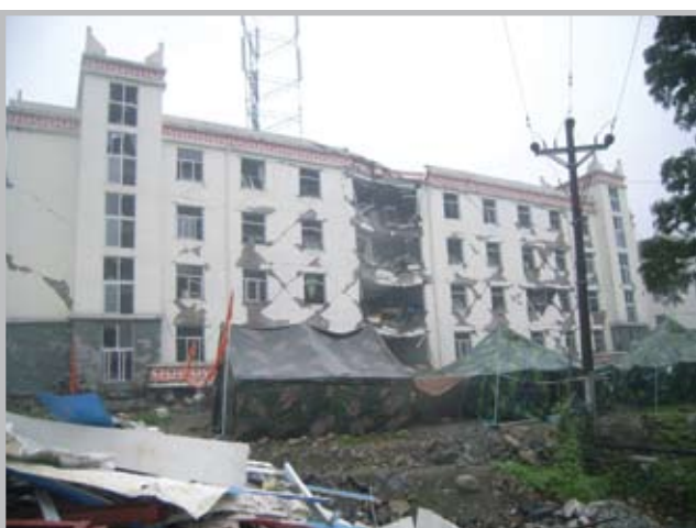
Partially collapsed five-story unreinforced masonry school building in Ying-Xiu (Source: EEFIT)
