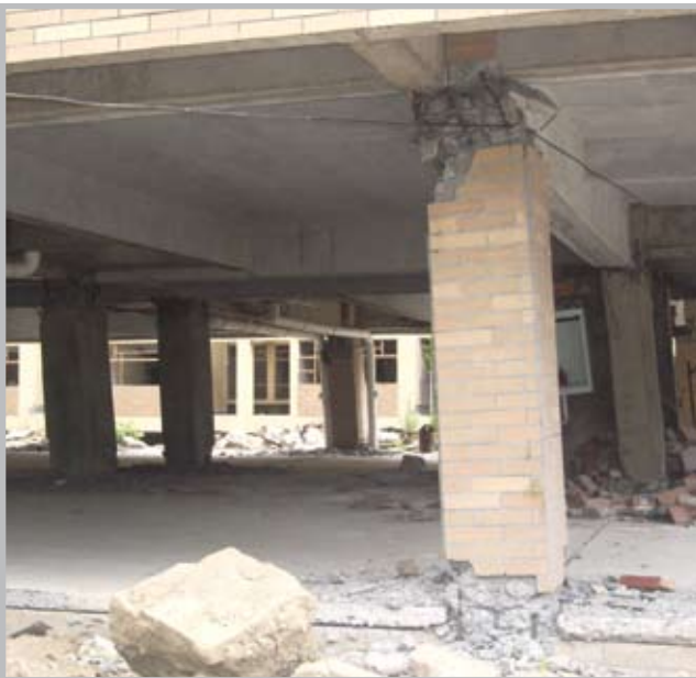
Soft-story failure of a six-story reinforced concrete residential building in Dujiangyan (Source: EEFIT)
