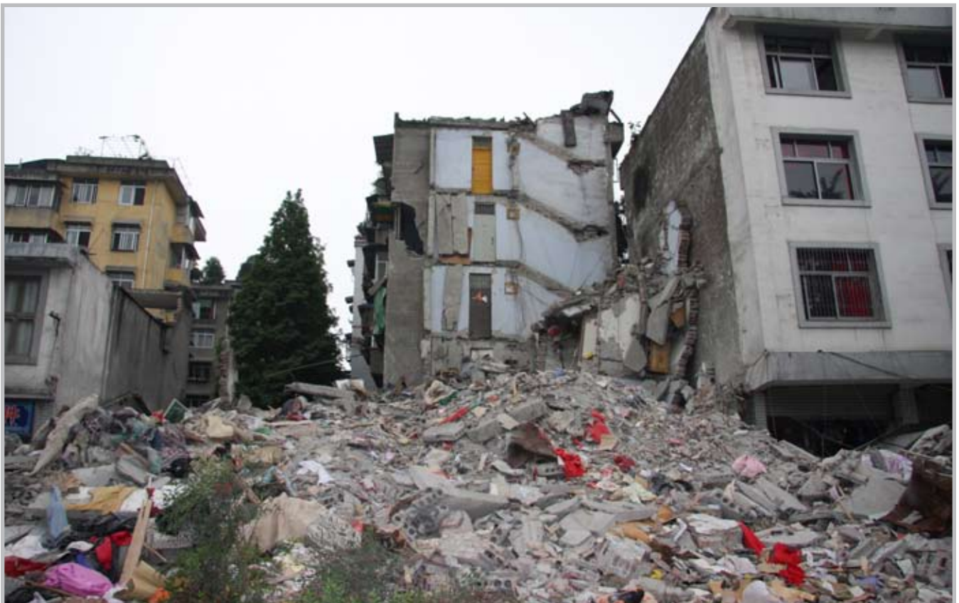
Differences in damage levels due to building age in Dujiangyan: The older building (center), designed with no seismic code, collapsed, while the newer building (right), designed to seismic code standards, remained intact (Source: IEM)
