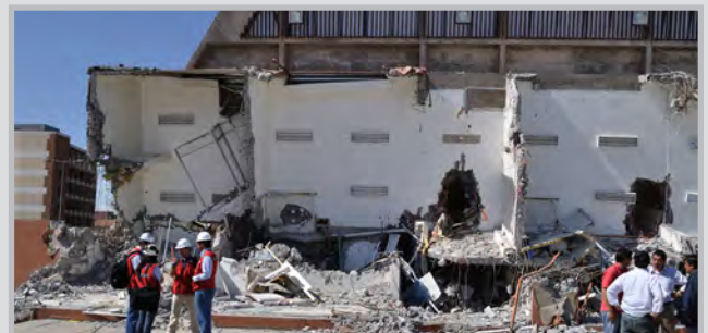
The west side of the Alto Río building, illustrating the slender shear walls at the ground level. (Source: RMS)
