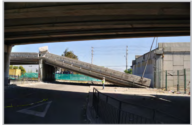
Collapsed span of the Autopista Vespucio Norte Express, connecting the Santiago International Airport to downtown Santiago (Source: RMS)
