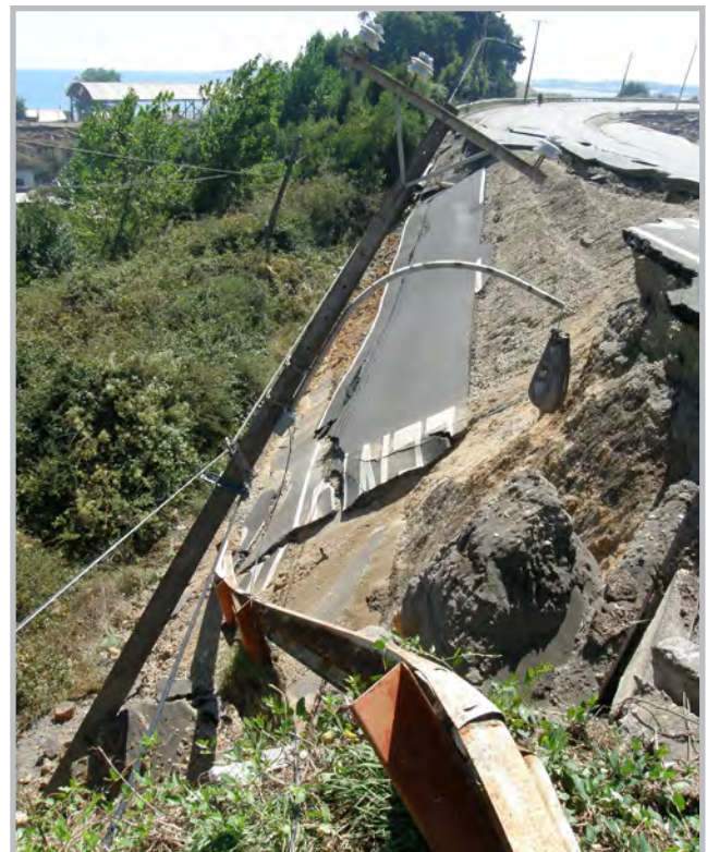
Failure of an overhead transmission line in Lota, Chile (Source: RMS)
