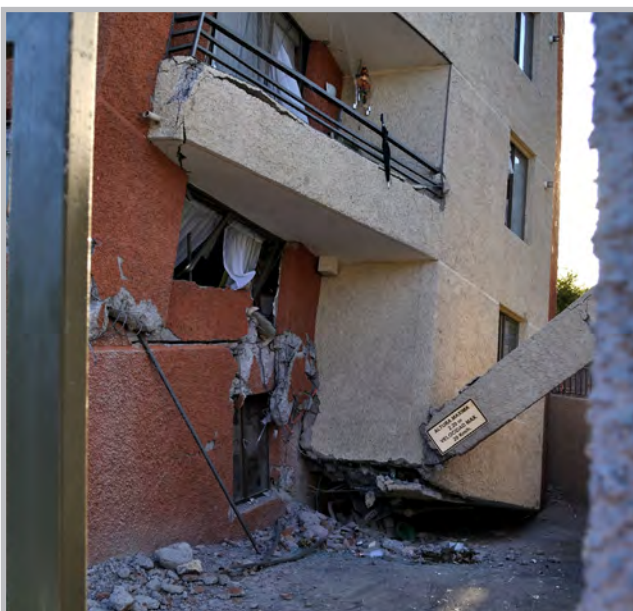
Soft story failure of a multi-family residential building in Maipú, Chile (Source: RMS)
