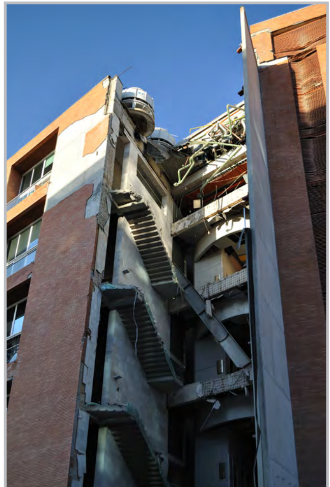
A building in the Huechuraba district of Santiago that sustained heavy damage as a result of ground motion amplification in the basin (Source: RMS)
