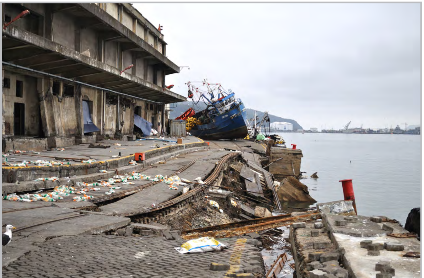
Destruction of the port facilities in Talcahuano, Chile (Source: RMS)
