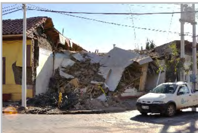
Collapsed adobe residential structure in Santa Cruz, Chile (Source: RMS)
