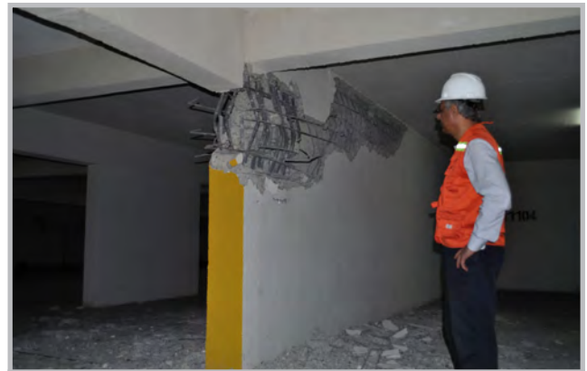
Shear wall failure observed in Viña del Mar, Chile, illustrating insufficient confinement and poor detailing of hooks (Source: RMS)
