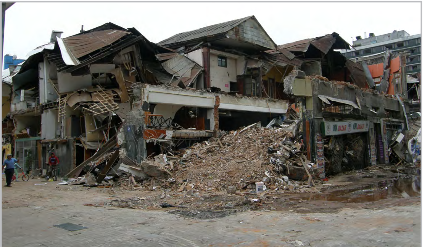
Collapse of low-rise confined masonry commercial structures in Concepción, Chile (Source: RMS)
