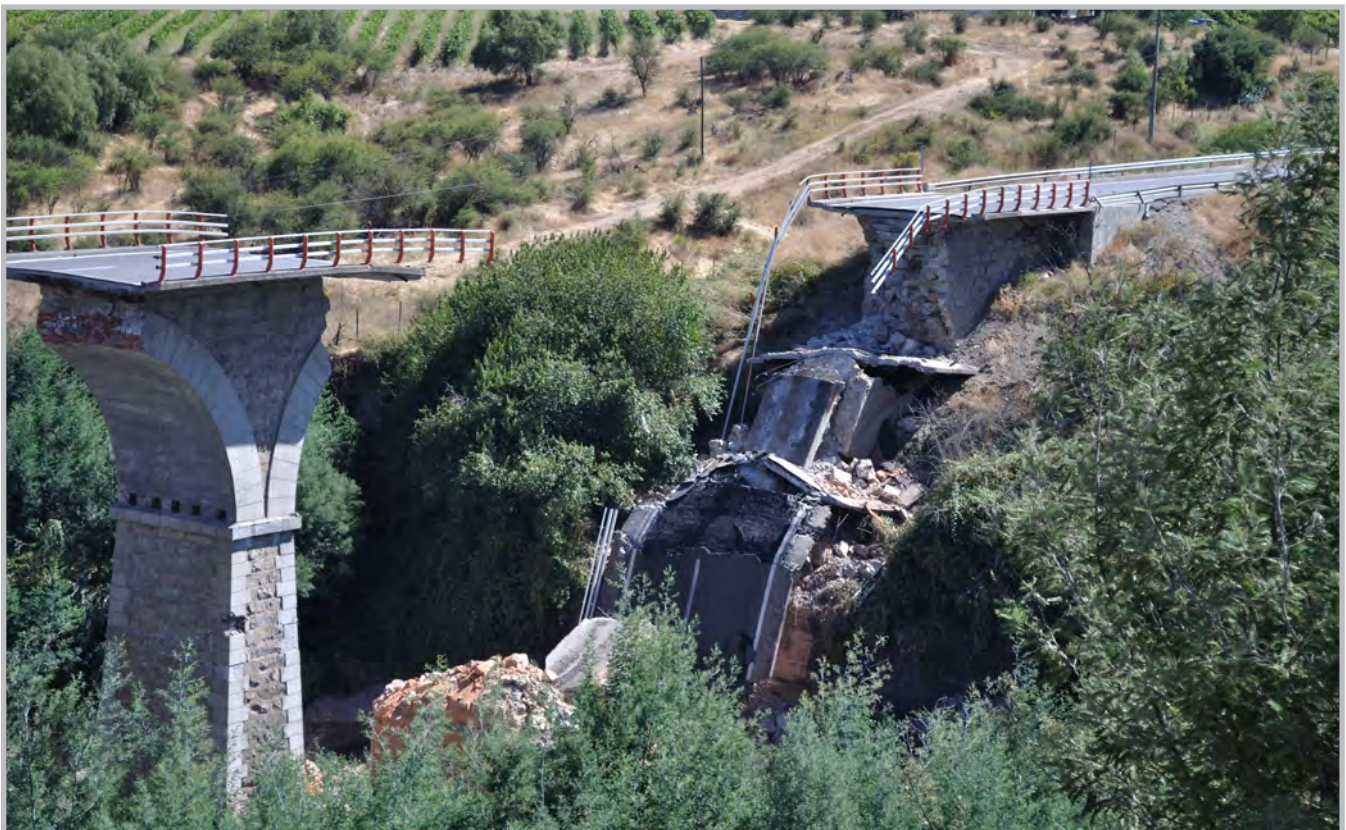
Collapse of an unreinforced masonry bridge, located between Curicó and Talca along Chile's Ruta 5 and spanning the Río Claro (Source: RMS)
