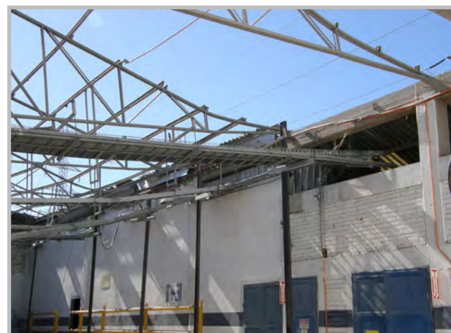
Light metal roof failure at the Inchalam wire manufacturing plant in Talcahuano, Chile (Source: RMS)
