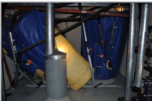
Overturning of a water tank on the top floor of an apartment building in Viña del Mar, Chile (Source: RMS)
