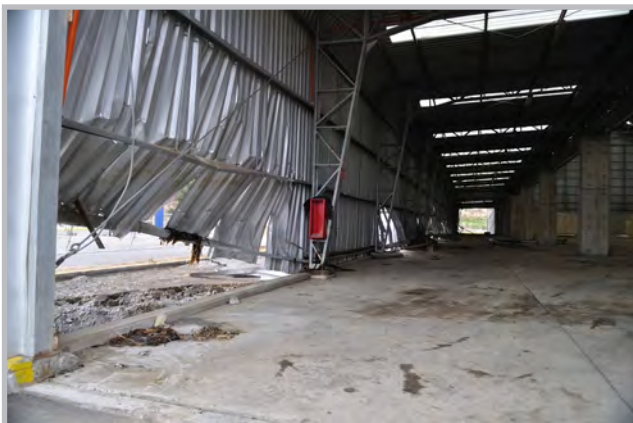
Tsunami damage in an industrial facility in Penco, Chile (Source: RMS)
