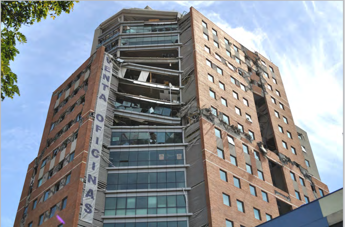
Partial collapse of O'Higgins Tower in Concepción, Chile (Source: RMS)
