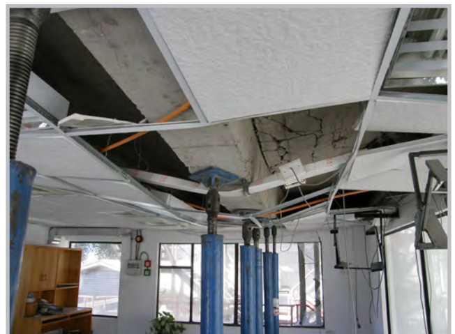
The cooling tower collapse (in picture above) caused the flexural failure of a beam in the operations unit of the Bío Bío cement factory in Talcahuano, Chile (Source: RMS)
