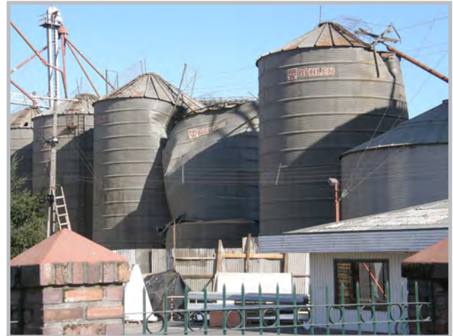
Failure of grain silos near Coronel, Chile (Source: RMS)
