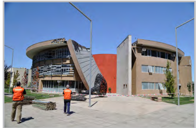
Damage to a chemistry building on the University of Talca's campus: a section of the roof detached from the wall and collapsed onto the walkway below (Source: RMS)
