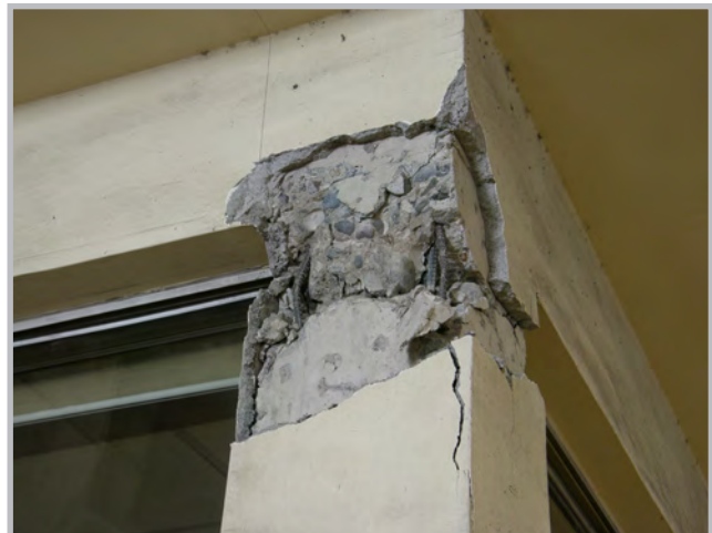
Failure of a reinforced concrete column as a result of lack of transverse reinforcement in the administrative office of the Inchalam wire manufacturing plant in Talcahuano, Chile (Source: RMS)
