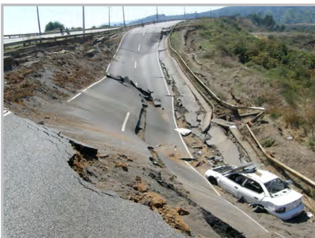
Damage to roadway near Lota, Chile following the 2010 Maule, Chile Earthquake (Source: RMS)
