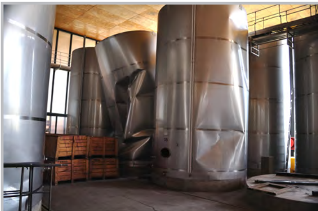
Damage to stainless steel storage tanks resulted in considerable amounts of contents loss to the Chilean wine industry (Source: RMS)
