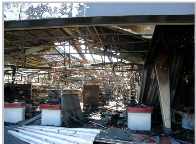
Grocery store in Coronel, Chile, destroyed by fire following the 2010 Maule, Chile Earthquake (Source: RMS)
