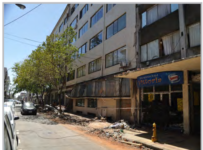
Damage to commercial buildings in Concepción, Chile (Source: RMS)
