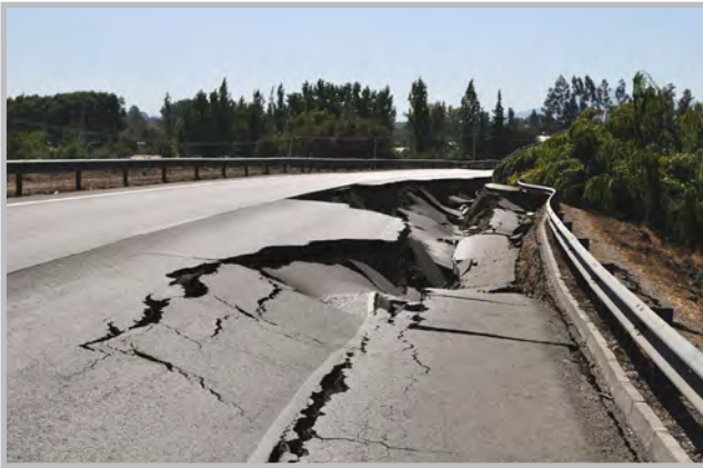
Buckled roadway along Chile Highway 5 (Ruta 5), south of Santiago (Source: RMS)
