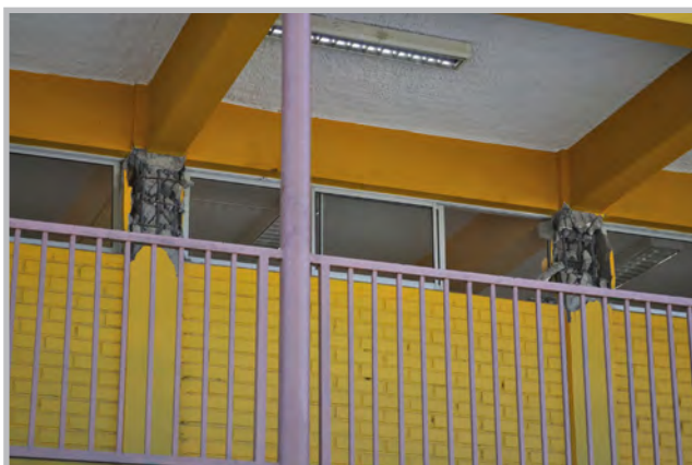
Damage to reinforced concrete “short columns” in a school building in the Santiago region (Source: RMS)
