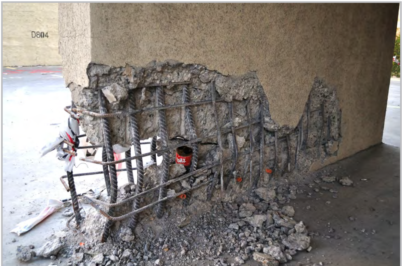
Damage in a tall apartment building in Viña del Mar, Chile; the shear wall failure was likely a result of poorly-detailed transverse reinforcement and insufficient wall thickness, as the concrete ruptured in compression and its longitudinal bars buckled (Source: RMS)
