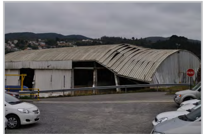
Observed damage to the Lirquén glass manufacturing facility in Penco, Chile (Source: RMS)
