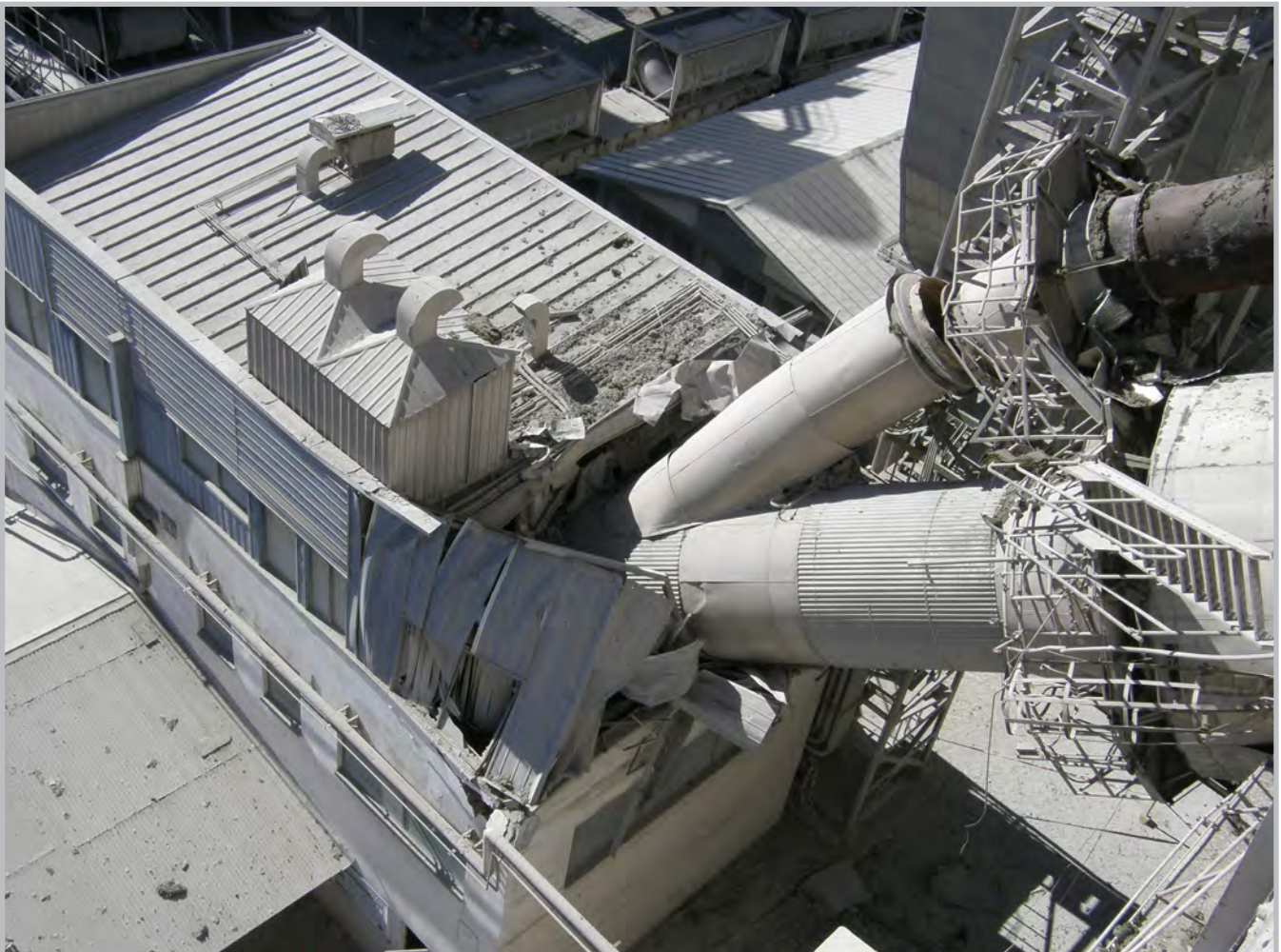
Collapse of a cooling tower at the Bío Bío cement factory in Talcahuano, Chile; fortunately, the failure of this tower did not impact the facility's production, as it was part of a backup system (Source: RMS)
