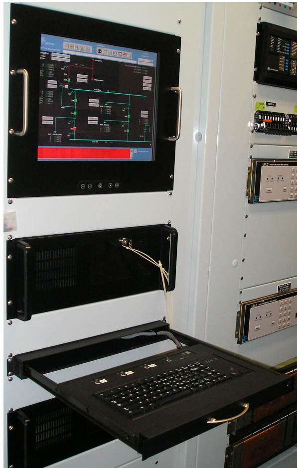
Figure 4 Substation Computer with HMI
