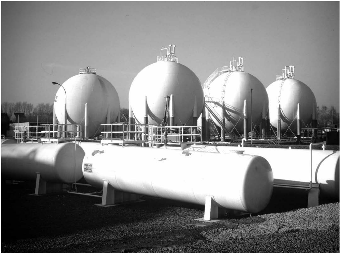
Fig. 31. Pressurized gas storage facility
