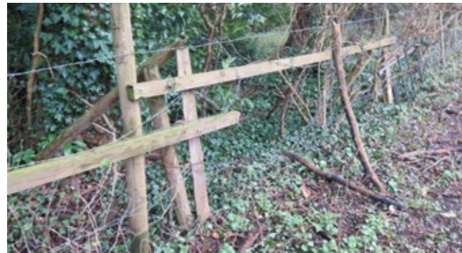
View of the state of the fence along the field edge of the wood
