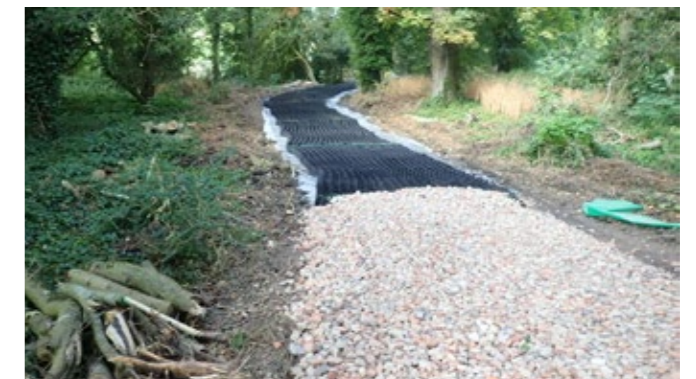
Construction through Wormstone Wood which lies in the Grade 2 listed Waddesdon Park - 2018
