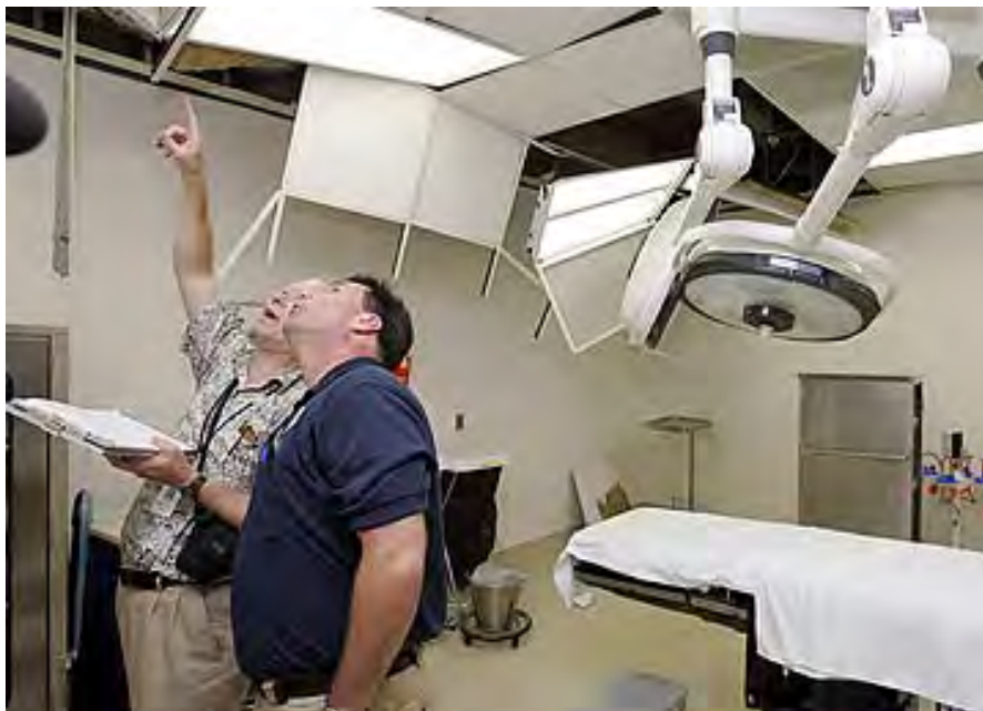
Inspecting damage to an operating room at a medical facility in Kona, Hawaii, after a magnitude 6.7 earthquake shook the region in 2006. [Photo by Mark Terrill, Associated Press.]
