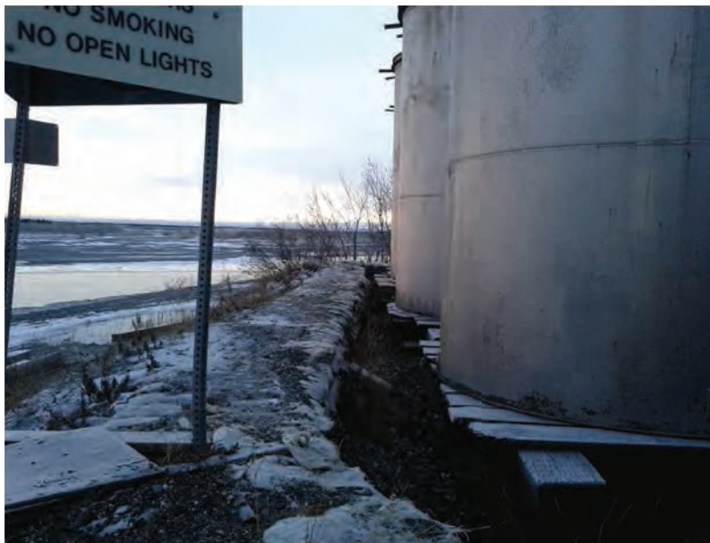
View of the diesel tank farm, retaining wall, and wooded plank support platforms. The Noatak river at lower water level is in the background. At high water level during spring melt, the river is within several feet of the tanks.
