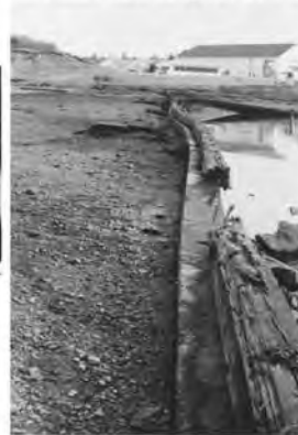
Seawall, Lateral Spread of Soil
