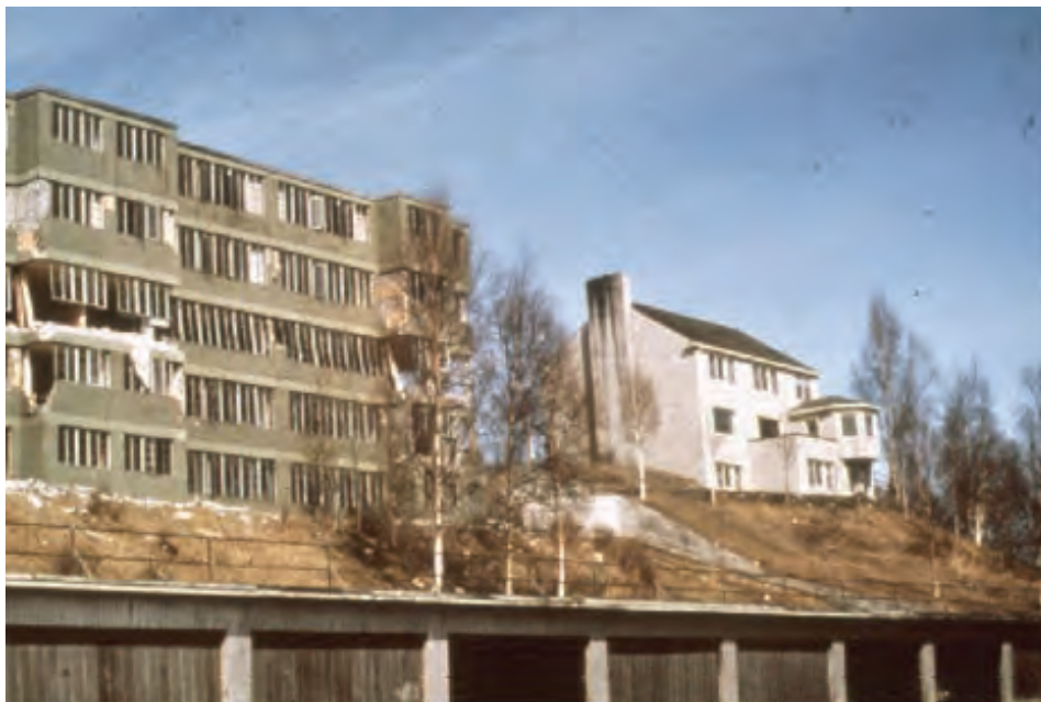
Damage to the concrete Hillside Apartment Building from the 1964 earthquake. Its wood-frame neighbor appears undamaged.
