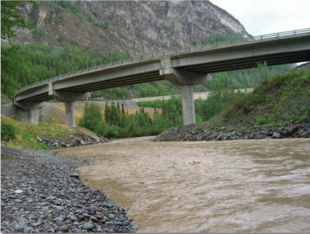
Caribou Creek Bridge, Glen Highway (less than a mile from the active Castle Mountain fault)
