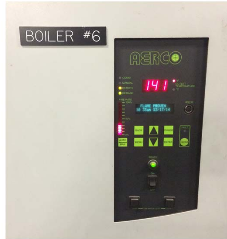
Photo 10: Burner Control Panel
