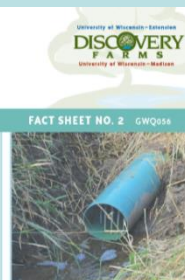
Figure 1: Tile outlet with a rodent guard.
