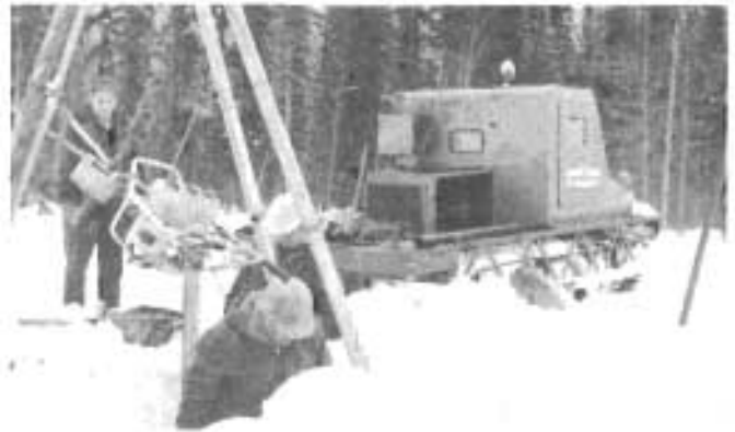
Materials testing crew installing deep settlement plates in a peat bog on the North Thompson Highway near Avola. Crew members are Don Garner, Dave Pecarski and Robbie Osborne.
