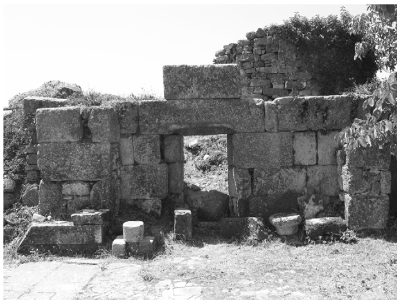
Fig. 17. The south wall of the church at Labraunda, originally belonging to the Roman East Bath. Notice the ashlar Pilasters 7 and 8 on either side of the entrance to Room 6.
