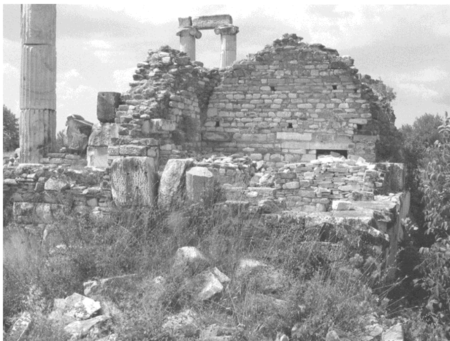
Fig. 18. Section of rubble wall (the north wall of the diaconicon ) in the Episcopal Church at Aphrodisias.
