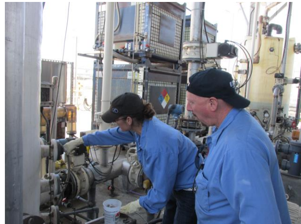
Figure 1: East Bay Municipal Utility District intern gaining hands-on experience with a journey-level Instrument Technician.
