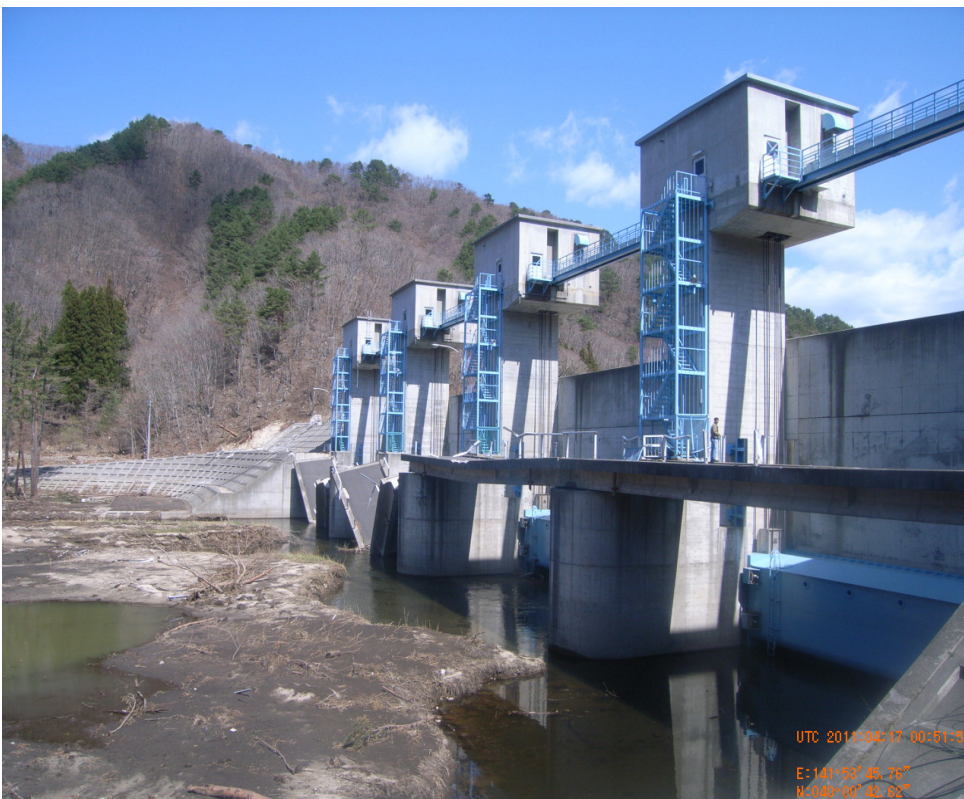
Seawall gate protected Fudai in Iwate Prefecture despite being overtopped. Photo courtesy of Gary Chock.
