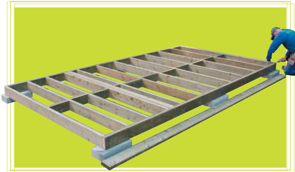
Designer and builder Wayne Lennox first constructed the Cottage Life Bunkie on site at the Spring Cottage Life Show. Here, he's prepping the double rim-joist floor framing.
