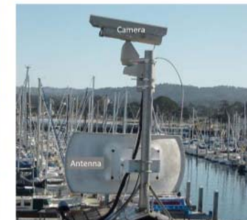
Fixed Transmit Antenna on Building Roof on Fisherman's Wharf
