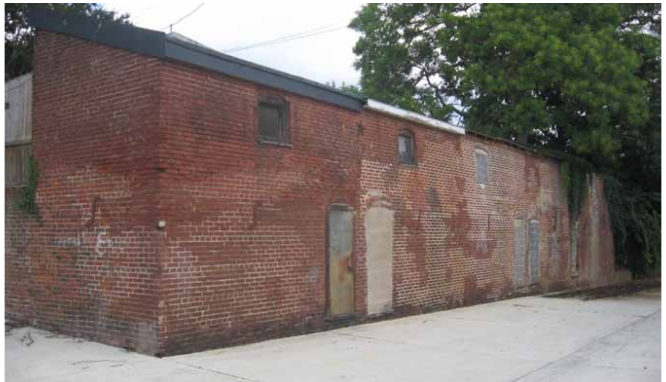
The two-story row of sheds at 611-619 G Street, SE date from before 1887, and are the oldest surviving sheds identified.
