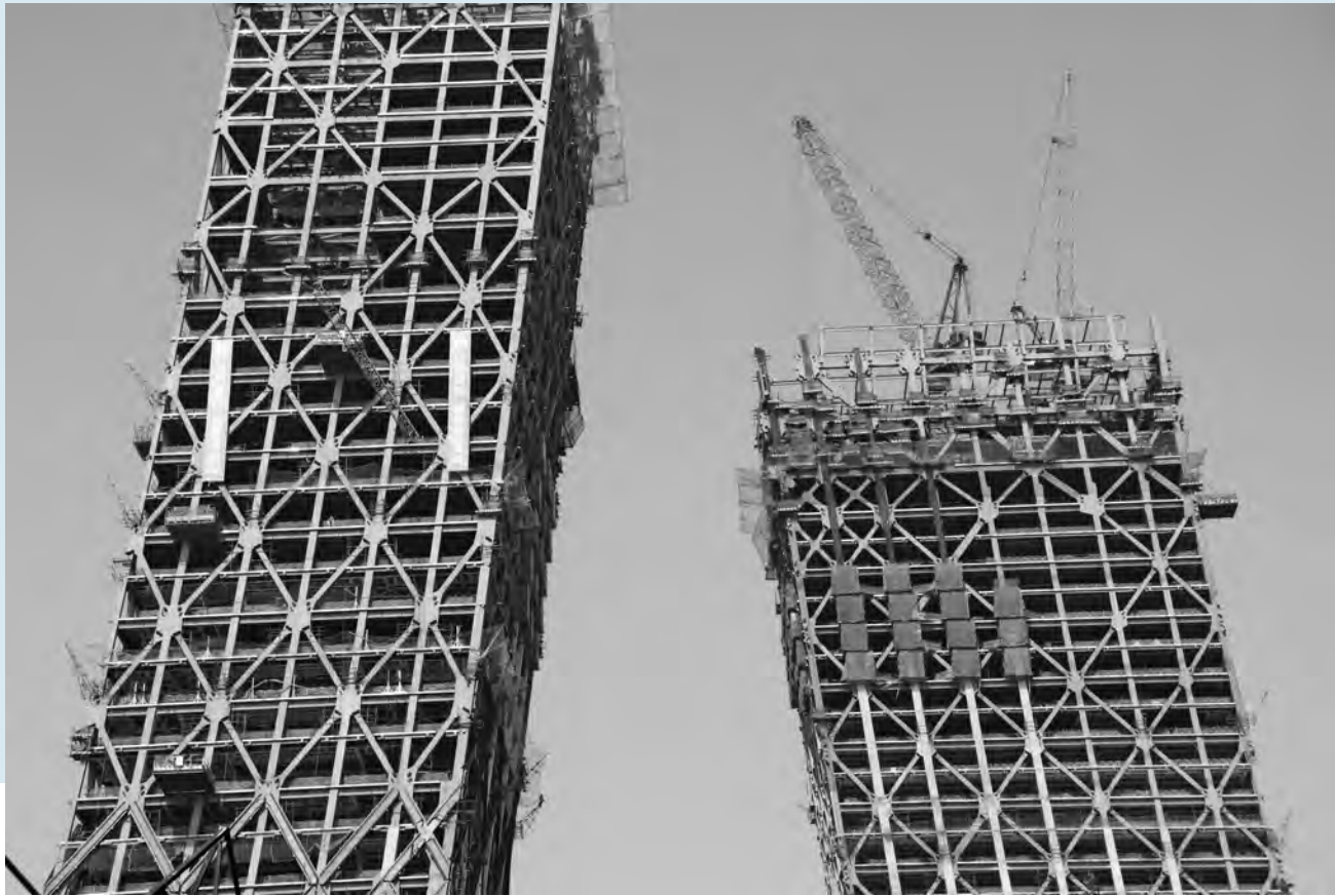
The diamond pattern framework of this high-rise building is used to resist loadings due to earthquake or wind.
