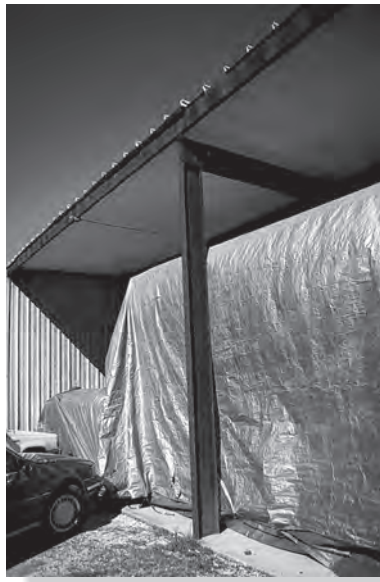
Wide-flange members are often used for columns. Here is an example of a beam column.
