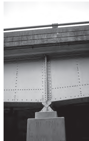
Typical pin used to support the steel girder of a railroad bridge.
