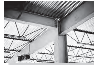
The two girders and floor beam are assumed to be pin connected to this column.
