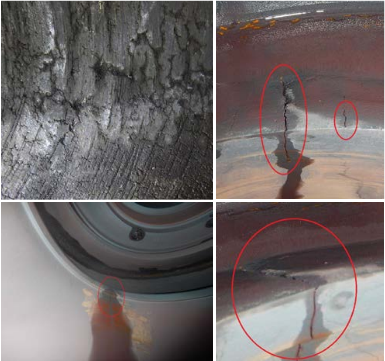
Figure 7-Cracks in BWCP pump cases
