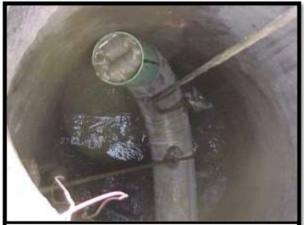
Excess CIPP Liner
