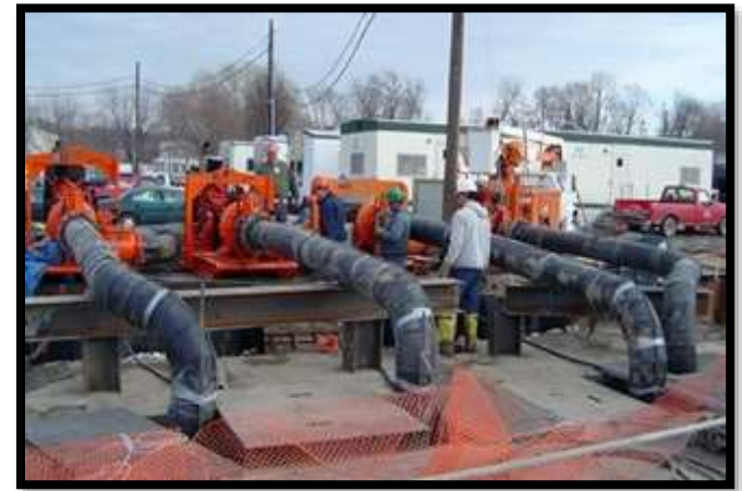
By Pass Pumping Equipment
