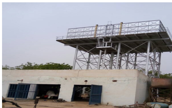
Rehabilitated Generator Room and 200m 3 Overhead Tank at Hadejia Main Pump House
