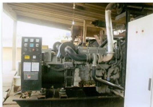
One of 6 Newly Procured 350 KVA Generator of Urban Water Schemes
