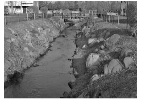
Penataquit Creek runs directly through Penataquit Village. The flooding has become so extreme that the water compromises the bank of the creek and even floods onto the nearby stretch of Union Boulevard.
