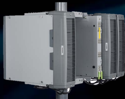
Cellular base station
