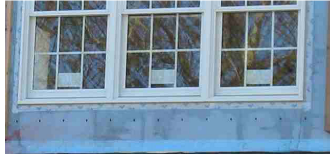
Figure 5 House during construction with water intrusion behind weather resistive barrier at window opening.
