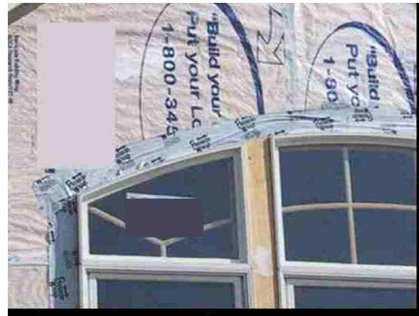
Figure 2 Rain has intruded directly through a perforated housewrap.
