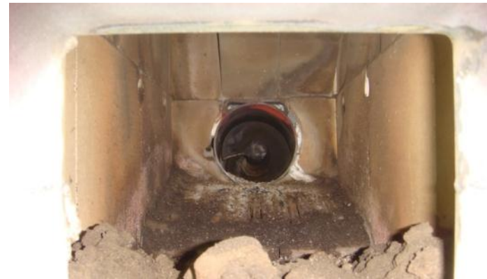
Moving Grate Primary Chamber Gasifies Pellets or Chips
