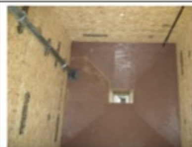
Pellet Storage In Pellet Hose Tower
