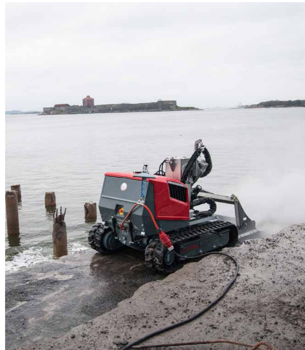
An Aquajet hydrodemolition robot in action at a berth in Gothenburg harbour.
