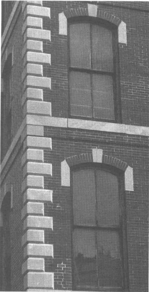
Figure 26. Decorative stone elements in the brick Greeley building, North Second and Lucas Streets. The large corner blocks and the window-arch "keystone" and "kneeler" blocks are Salem Limestone ("Indiana Stone"). Photo by Art Hebrank.
