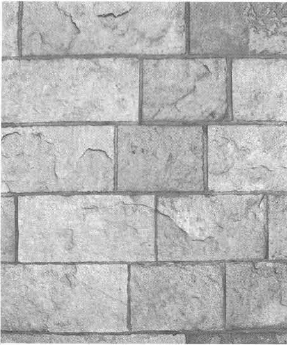
Figure 3. Ashlar masonry facade of the Old Cathedral. The dolomite ashlars are about one foot high. This is called coursed ashlar masonry--all blocks in any one course are of equal height. Photo by Art Hebrank.
