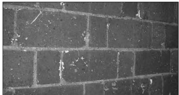
Damage to brick surface as a result of inappropriate sandblasting
