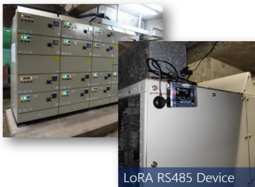
Fig. 5 - LoRa RS-485 device installed at swimming pool filtration system
