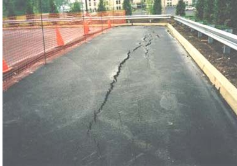
Fig. 13 Tension cracks occurring exactly at the end of the wall reinforcement (authors)
