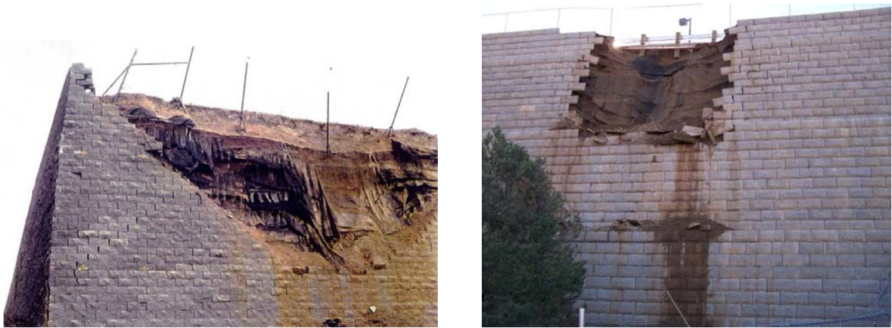
Fig. 6 Cases of wall collapse (various contributors including authors)
