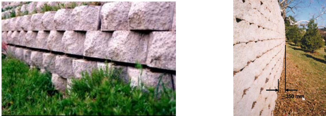
Fig. 5 Cases of excessive wall deformations (various contributors including authors)
