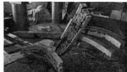
Curved members, such as stemhead and stern knee, are built up of laminates.
