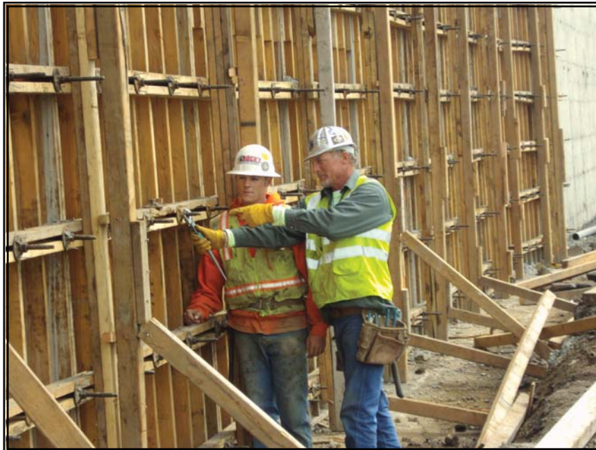
Apprentice Matthew Kunz (L) gets some bridge building tips from foreman Rance McFarland
