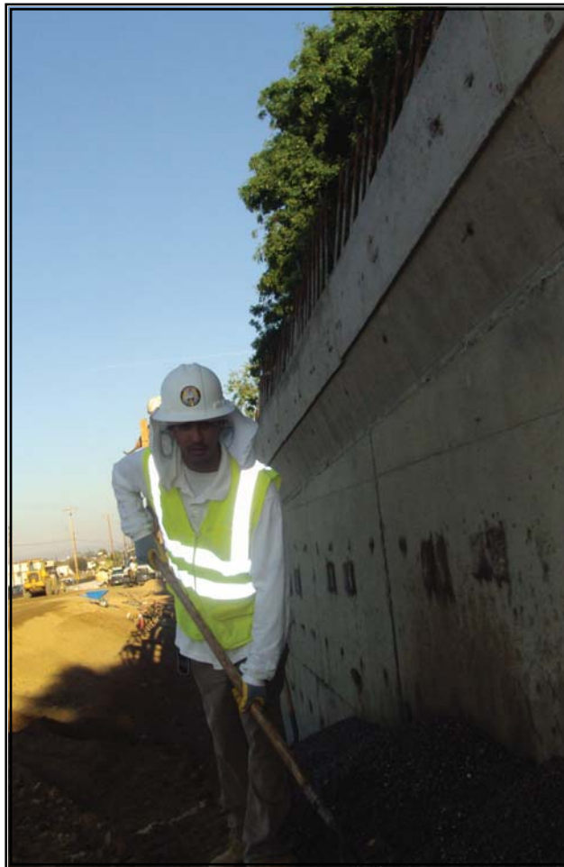
Apprentice Jose Madrigal hard at work on the Highway 99 overpass project in Ceres.
