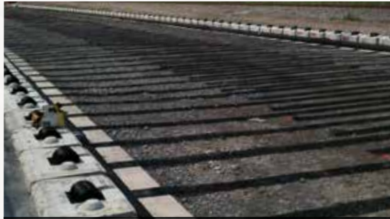
The Canadian National Railway used PC System walls in Montreal to elevate a rail line. These walls are engineered to withstand extreme live loads. See page 10 for more on this project.
