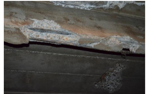
Damaged Concrete & Exposed Reinforcement in Joist
