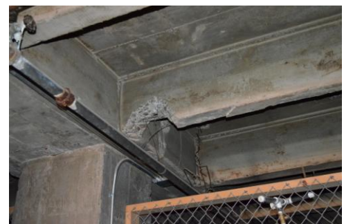
Damaged Concrete & Exposed Reinforcement in Joist
