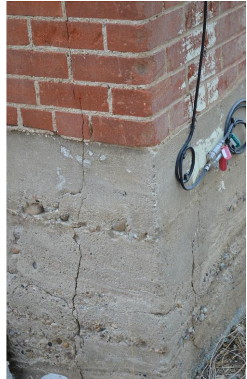
Example of Visible Cracking in Foundation Wall
