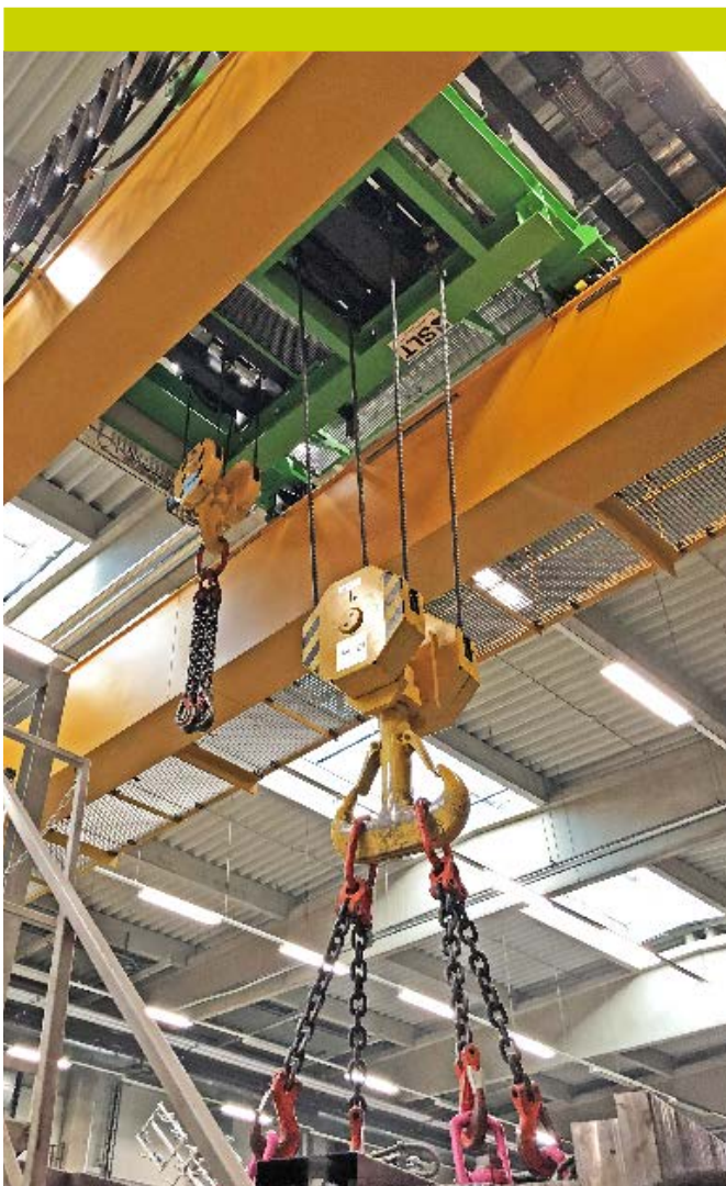
A new travel carriage with an ASF7 as main and an SHF6 as auxiliary hoist was installed on the existing double girder overhead travelling crane.
