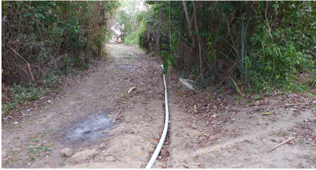
Figure 7. The plastic tube is shown that is used to protect the power supply and fibre optics cable running from the electronics house (visible at the far end in the image) to the variometer house (not visible).
