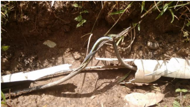
Figure 11. The power cable between the variometer house and the electronics house was damaged a few metres from the variometer house due to currents induced by a lightning strike close to Tatuoca observatory on 31 December 2016.
